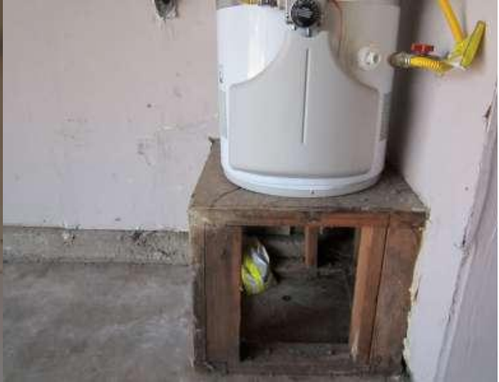
Photo 35 Support box needs to be better supported (i.e. repaired and leveled) or replaced.
