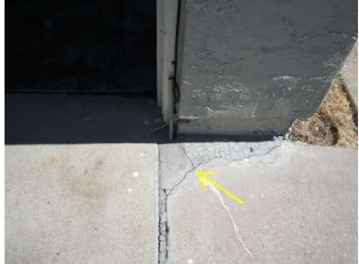
Photo 40 Former repair. Vinyl patching like this will need to be replaced every 7 to 10 years.
