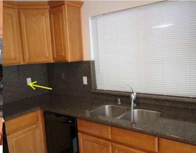
Photo 21 Needs to be a GFCI.
