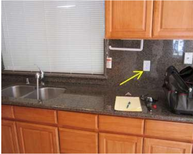
Photo 20 Needs to be a GFCI.
