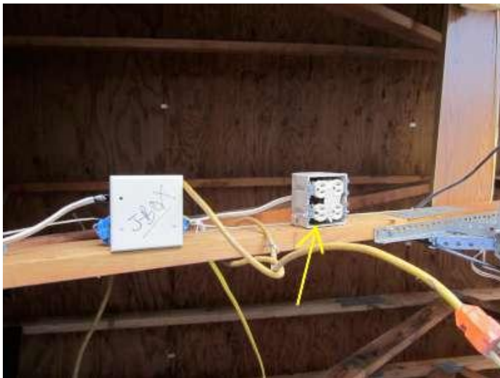
Photo 38 Cover plate needed.
