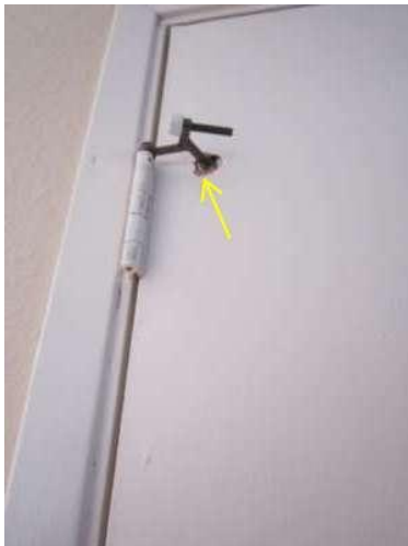
Photo 27 After door is repaired or replaced, if this or a similar piece of hardware is installed, I recommend installing a metal base place at the location of the arrow.
